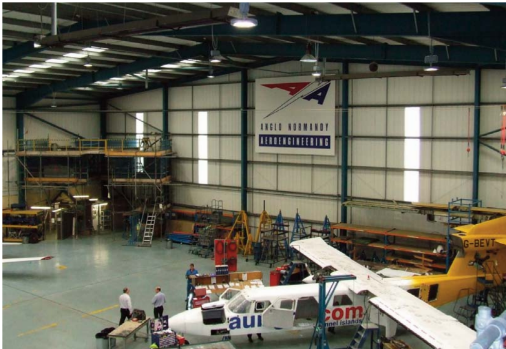
Lit by Dialight's 250W LED high bays the hangar now achieves 400 lux at work height
