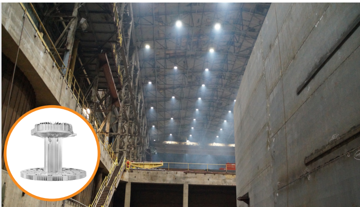
Dialight Vigilant® 60,000lm LED High Bay Fixtures cut through the dust at Donjon Shipbuilding and Repair
