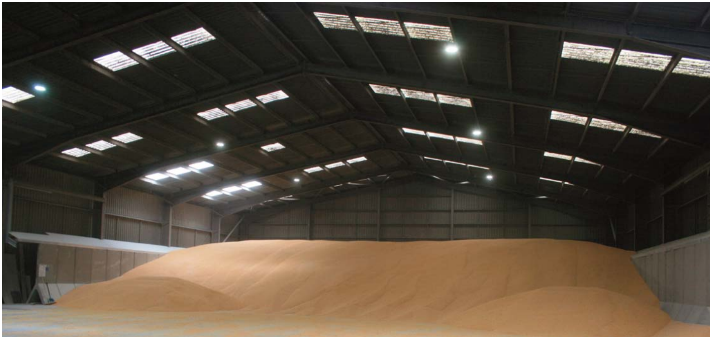
Shed 3 lit by eight of Dialight's 172W LED high bays
