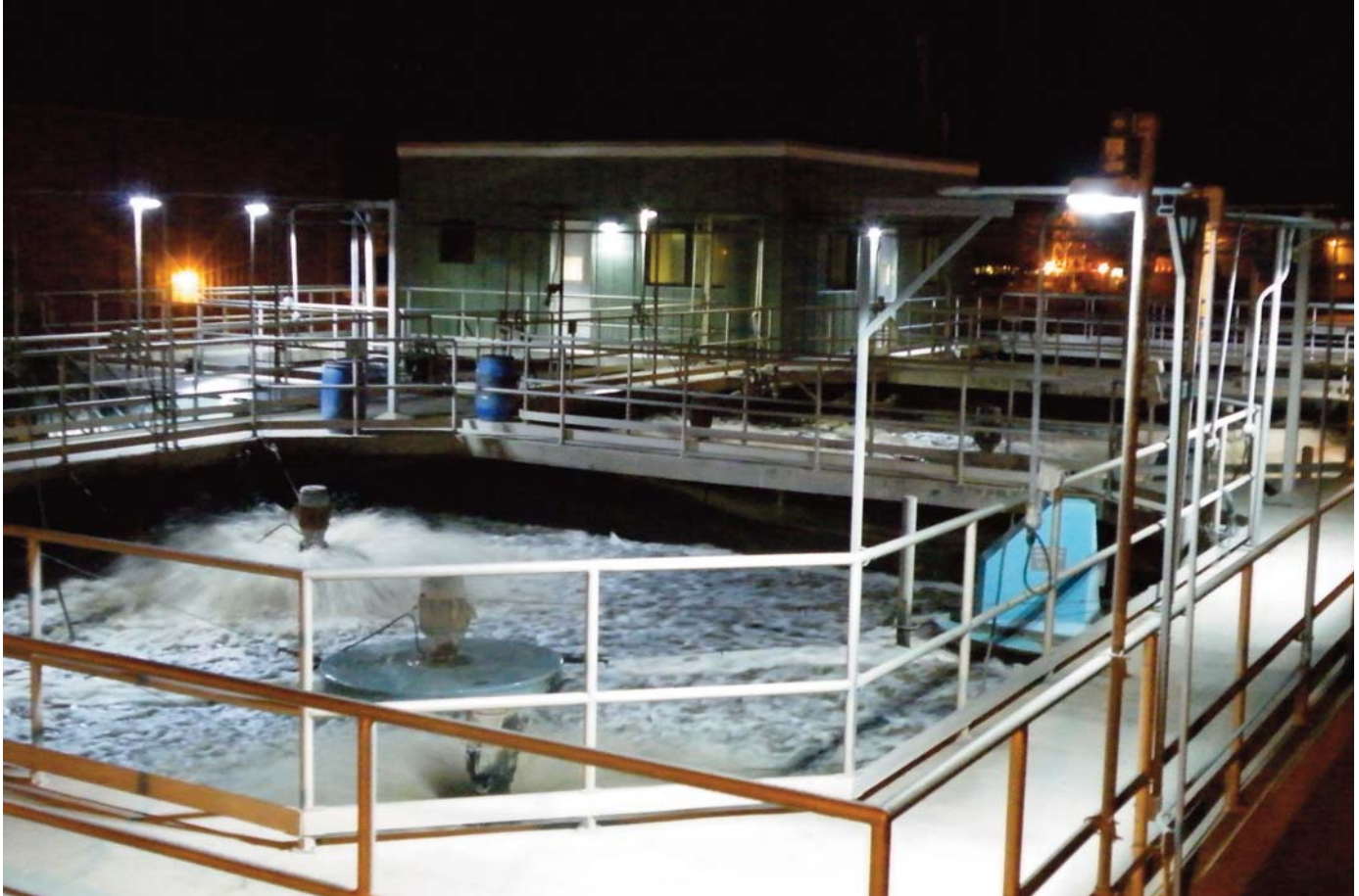
New SafeSite® LED lighting in the foreground and HPS lighting in the background.
