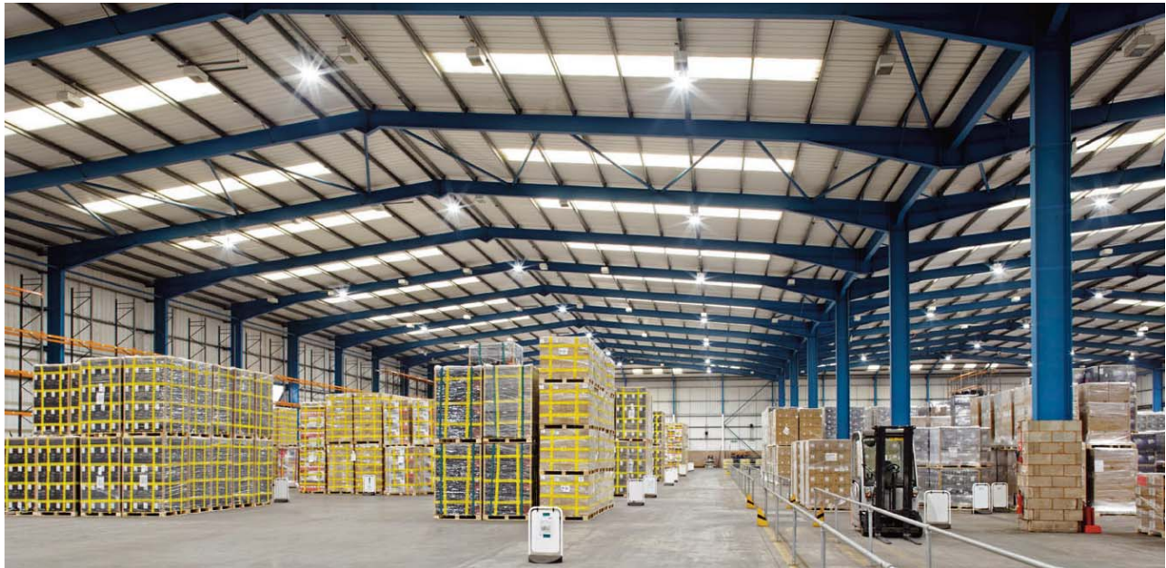
Dialight's DuroSite™ Series LED High Bay Fixtures Installed in Kuehne + Nagel's Minworth warehouse
