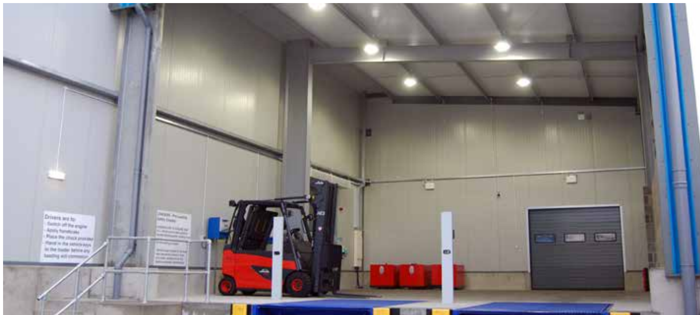
Dialight DuroSite® LED High Bays with Instant on switching allows MMD Shipping to achieve even greater savings
