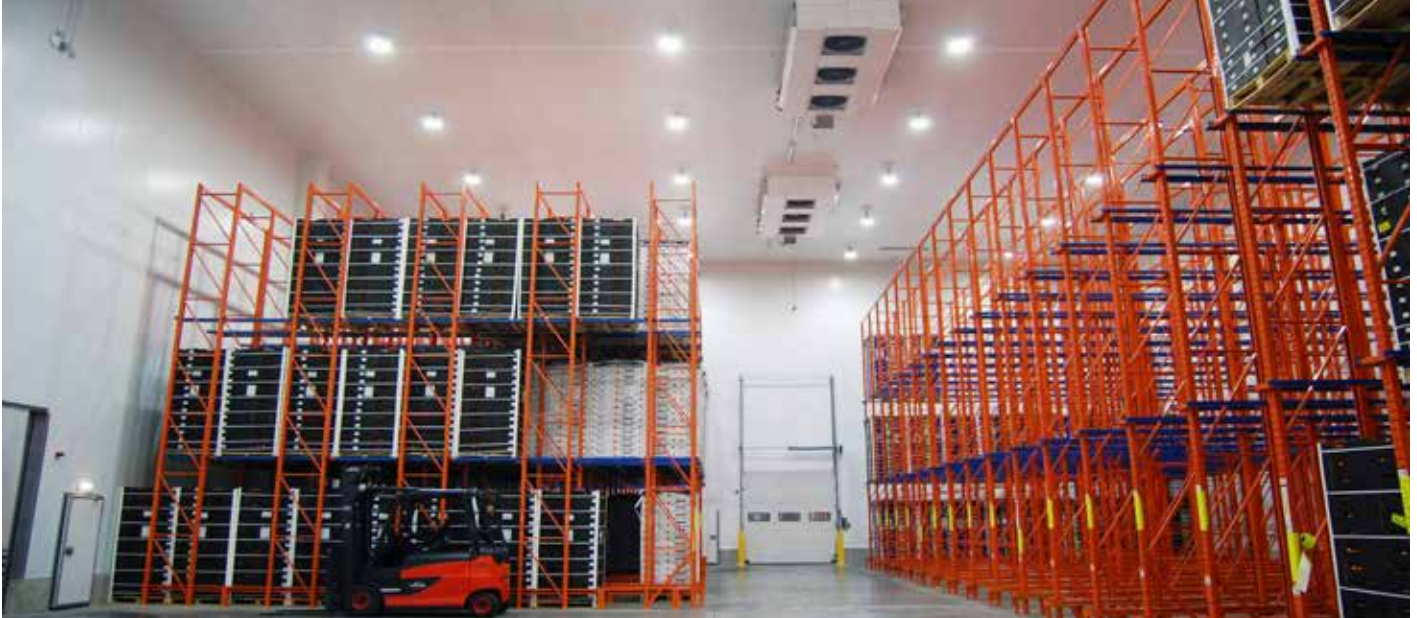
Dialight's DuroSite® LED High Bay fixtures installed in MMD Shipping's Portsmouth ware-
