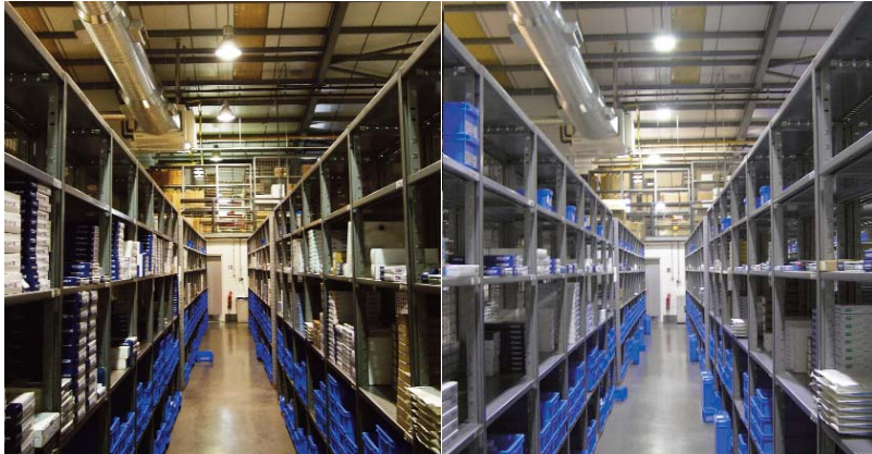
Olympus KeyMed warehouse lit by metal halide on left and then by LED on right.
