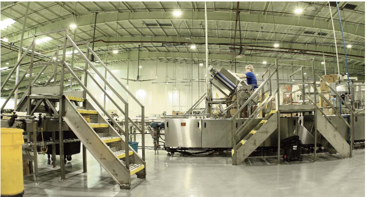
Dialight's DuroSite™ Series LED High Bay Fixtures Installed in Rockline's Booneville, AR production facility
