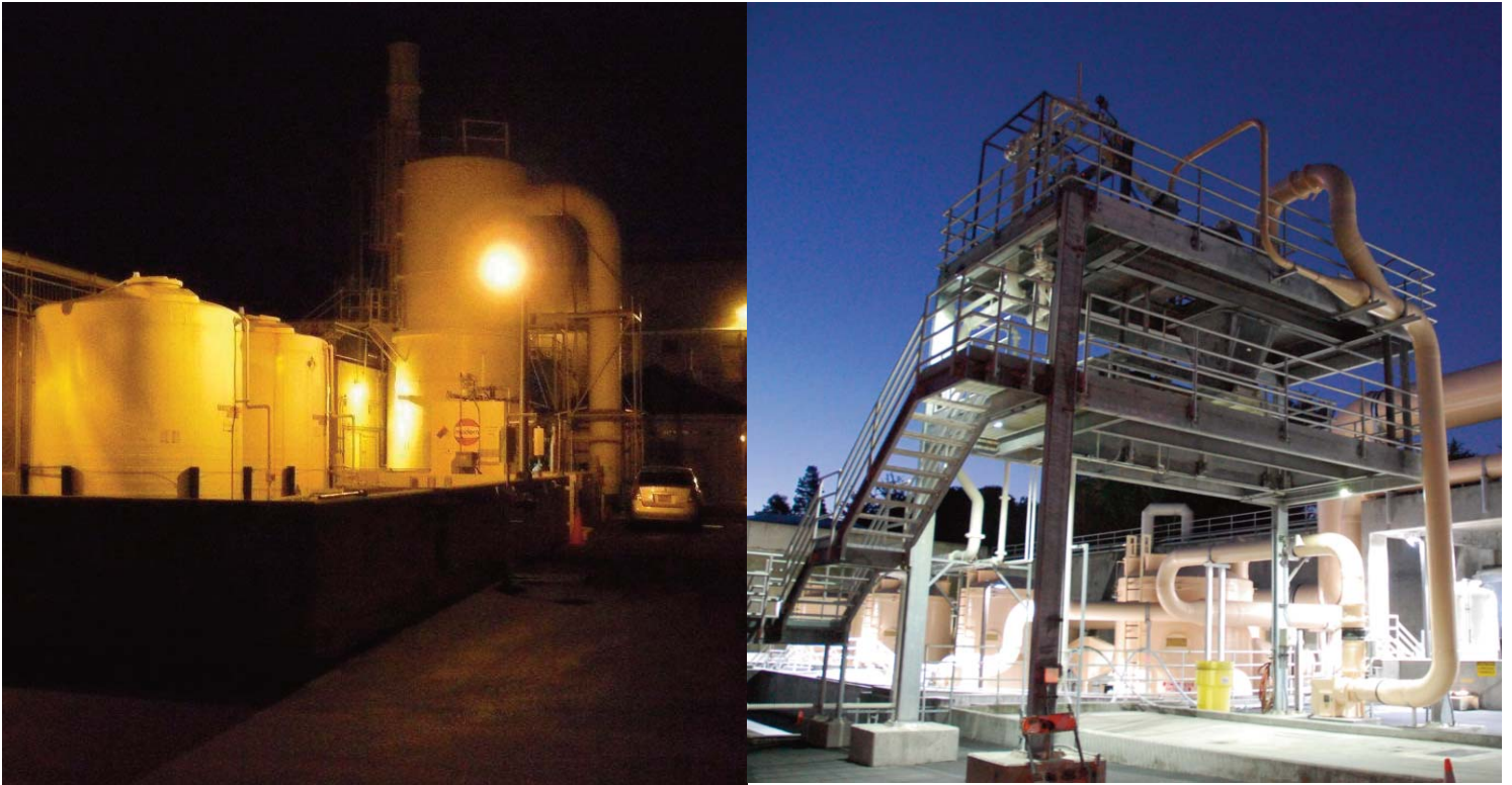
High pressure sodium fixtures previously installed at Santa Cruz WWTW provided poor quality of light. Dialight's LED lighting fixtures not only provide improved light quality, they also slash energy and maintenance costs
