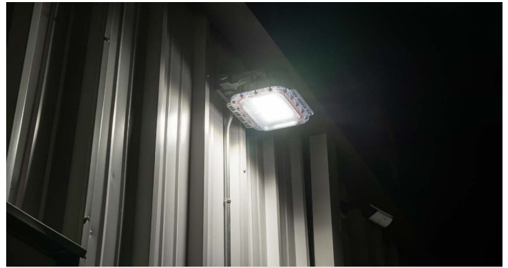
Dialight LED Area Light at Gas Monkey Garage.
