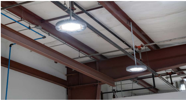
Dialight LED High Bays in the Gas Monkey Garage Man Cave.
