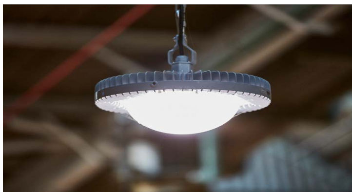
Dialight Vigilant® LED Low Bay installed at D.S. Smith.
